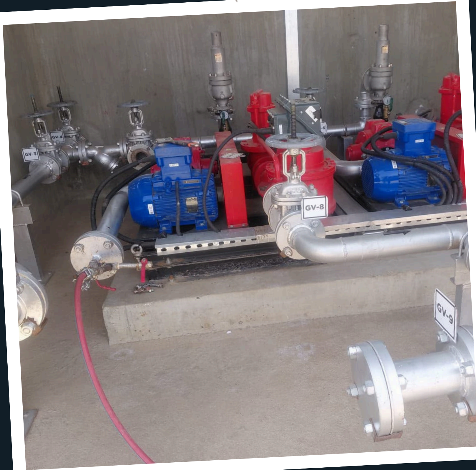
INSTALLED FUEL PUMPS
